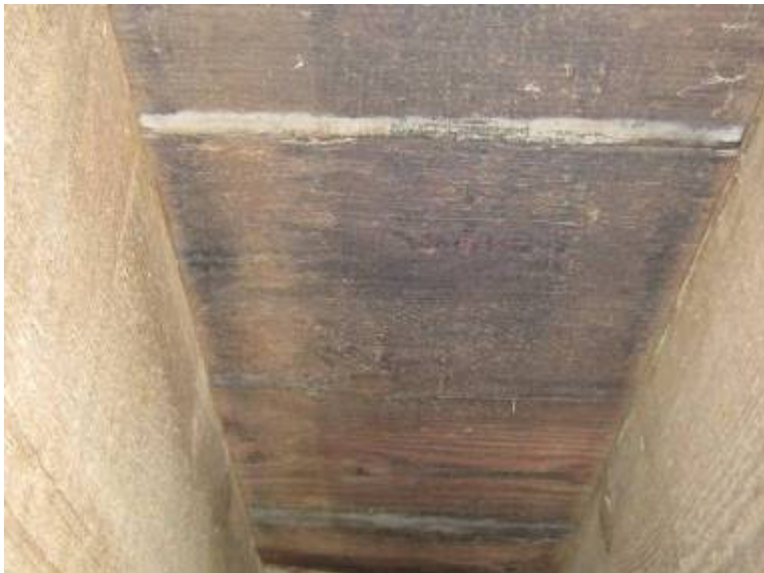
Figure 4-40. Underside of deck in good condition with no visible defects or bleeding
