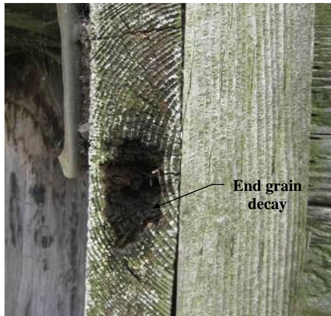
Figure 4-15. Poor end grain with decay was most common defect found in backwalls.
