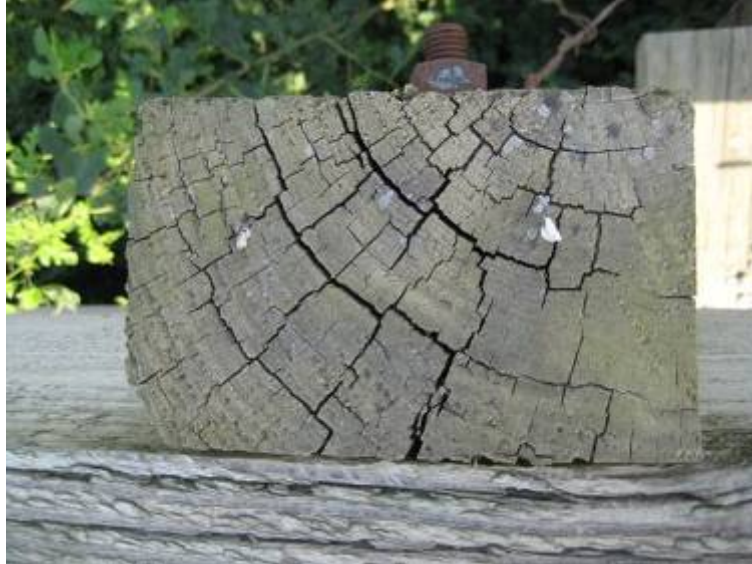
Figure 4-57. Top of a guard rail post showing end grain physical defects
