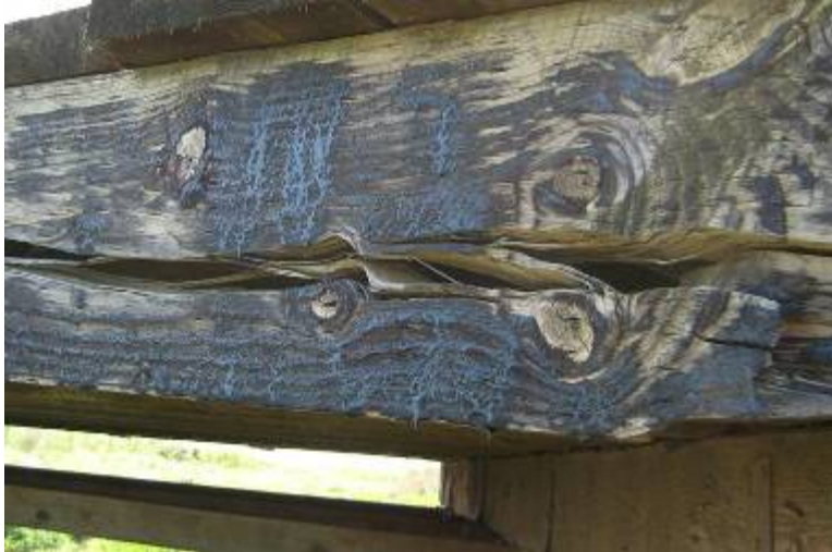
Figure 4-22. Poor exterior stringer with creosote bleeding and severe split.
