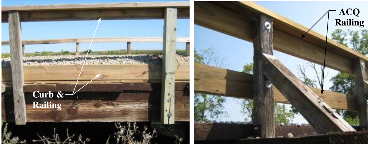
Figure 4-60. ACQ treated lumber used as guard railing members
