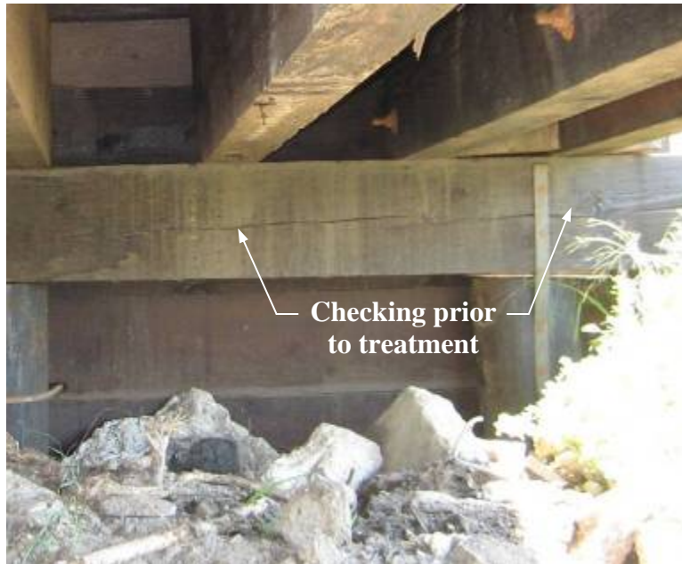
Figure 4-31. Good cap beam with seasoning prior to treatment allowing preservative to infiltrate longitudinal checks creating a complete preservative barrier
