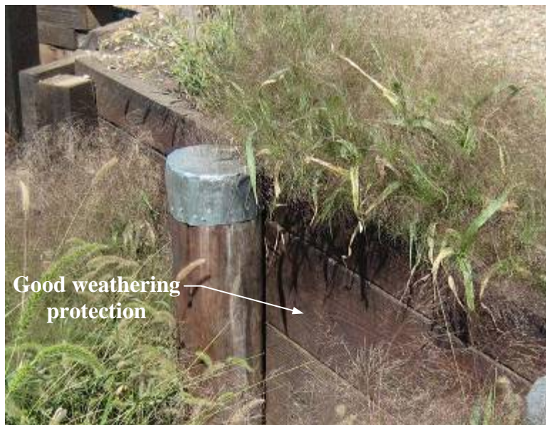
Figure 4-33. Good wingwall with very little ultraviolet degradation and no treatment bleeding.
