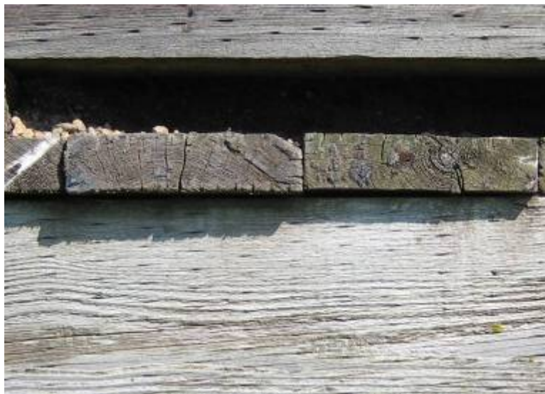
Figure 4-42. Physical defects at endgrain, ca. 1980
