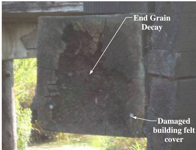
Figure 4-12. Poor pile cap with exposed end grain and decay
