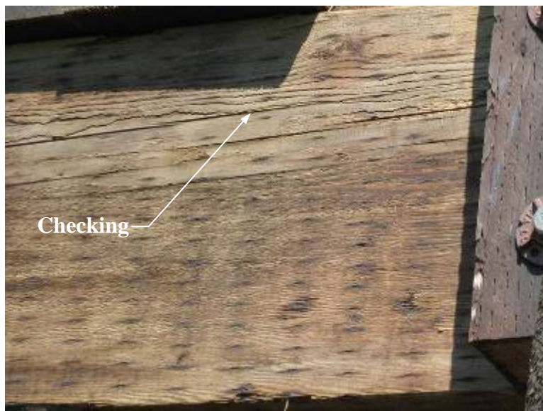
Figure 4-38. New exterior string with seasoning checks forming on the surface
