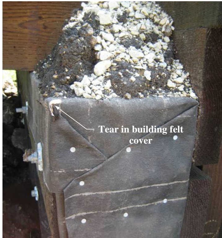
Figure 4-46. End of pile cap with building felt cover providing protection from moisture and weathering
