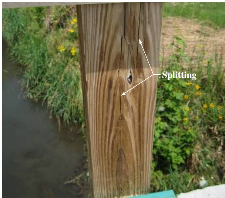
Figure 4-61. ACQ railing post with splitting that is generally associated with waterborne treatments
