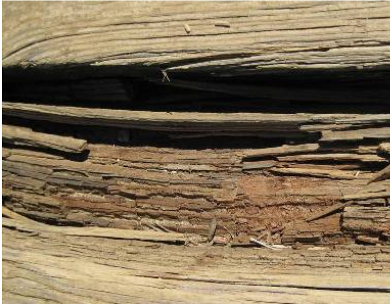
Figure 4-27. Pooling water allowed brown rot to grow on mechanically damaged deck surface
